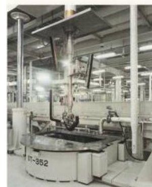
▲Tank washing station
