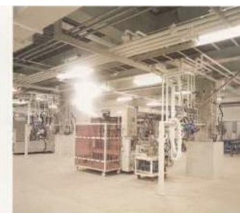
▲Filling facility at the 1st FL
