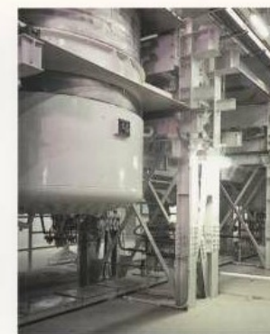
▲Vessel in the station
